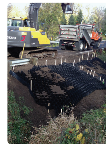
Flooding in 2012 in Northeast Minnesota damaged roads and bridges, water and sewer systems and other infrastructure, costing $108 million. More than 1,700 homes and 100 businesses were damaged or destroyed, costing more than $12 million.
