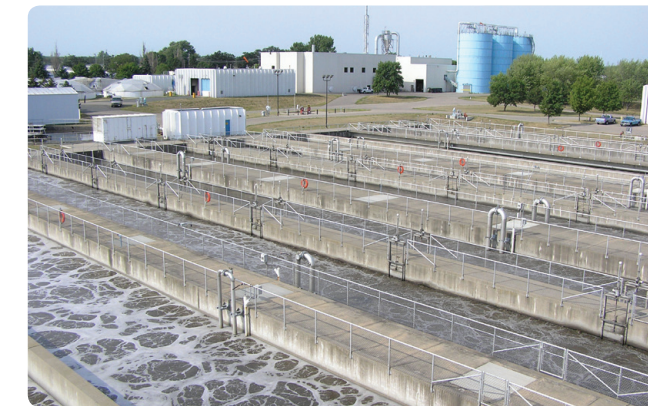
The Blue Lake wastewater treatment plant treats an average of 29 million gallons of wastewater per day.
