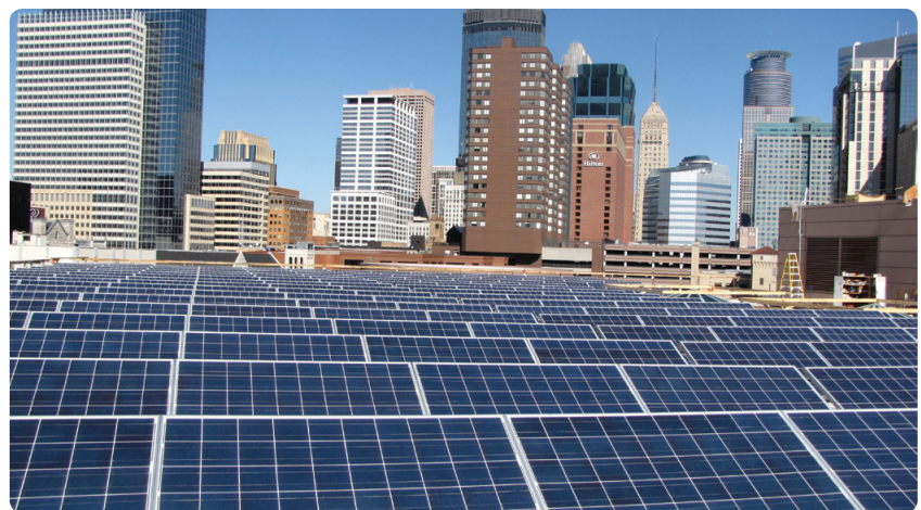
More than 2,600 solar panels sit atop the Minneapolis Convention Center and help directly power the facility. (Photo Credit: Minneapolis Convention Center)
