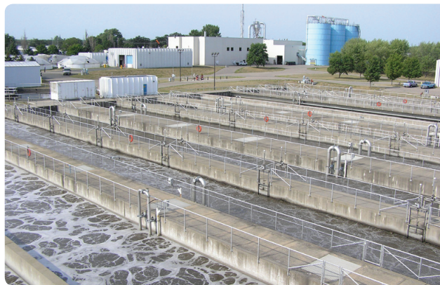
The Blue Lake wastewater treatment plant treats an average of 29 million gallons of wastewater per day.
